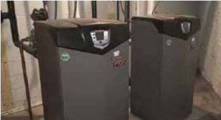
These are the new hot water boilers which now provide heat inside the church.
